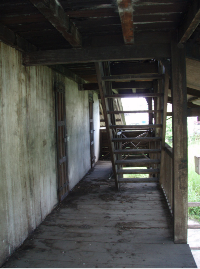
Rotten timber floorboards and staircases, before restoration.
